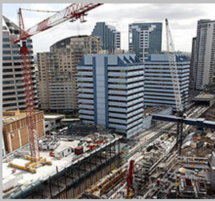
Aerial view of the construction works at the Chatswood Transport Interchange site
