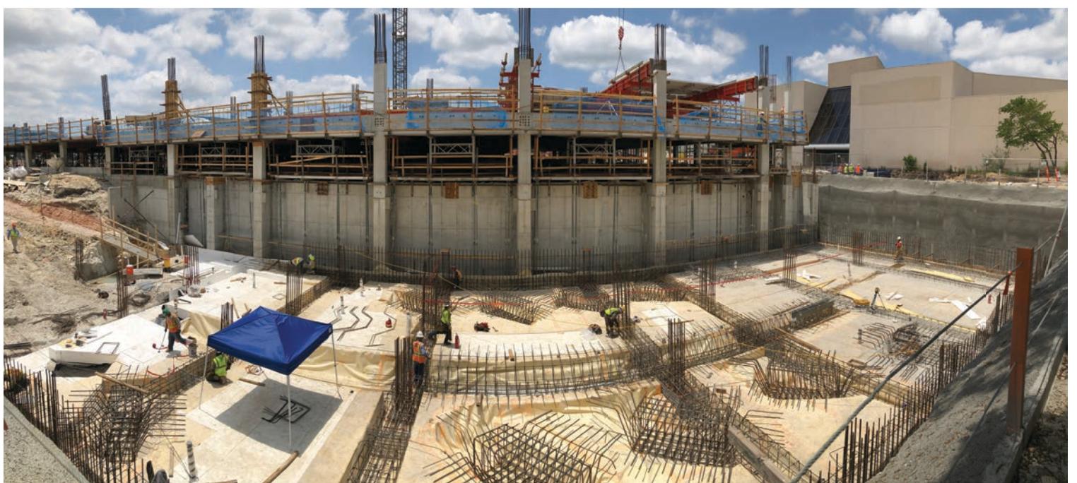
Hydrostatic pressure challenge: Plans called for the chiller plant to be built about 20-feet (6 m) below-grade, making a robust waterproofing solution an important part of the project specifications.
