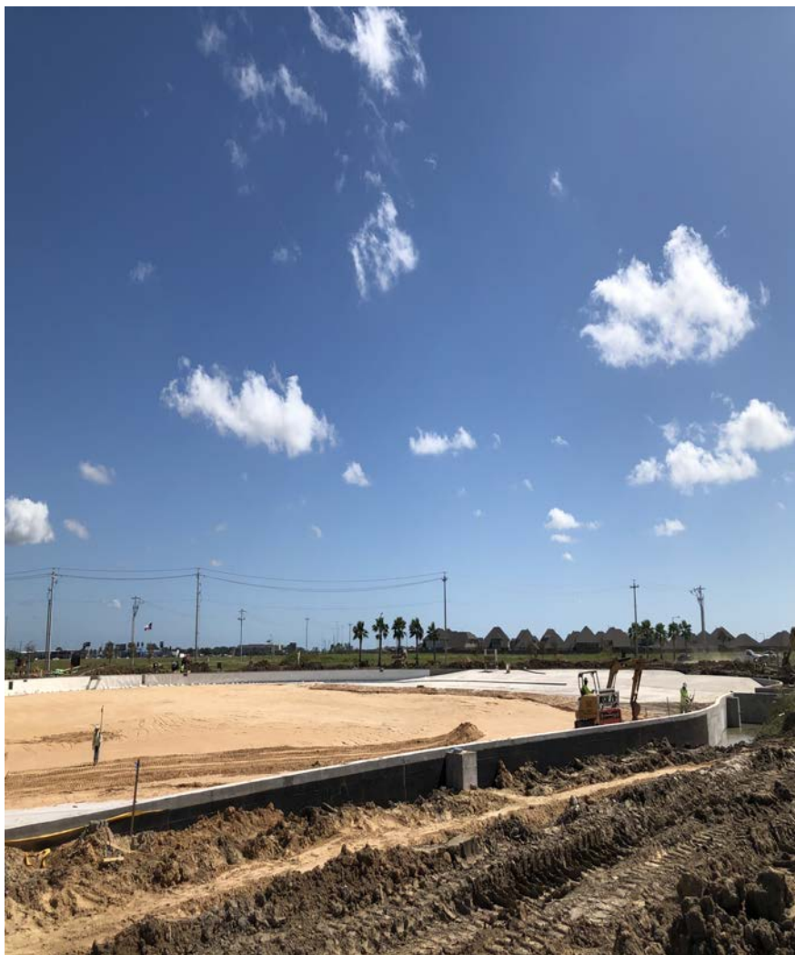
Just add white sand: PENETRON slurry was applied to the surface of the Crystal Lagoon's beach area (in Texas City) to help prevent water penetration into the concrete structure.
