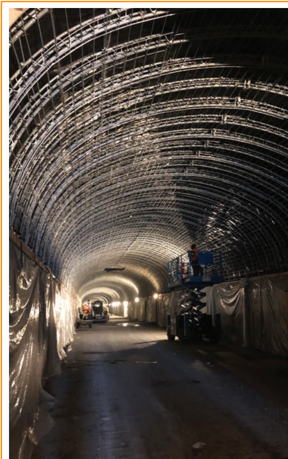
A crystalline solution: Originally built in the mid-1800s, the structural remediation of New York's Park Ave Tunnel (1,600-foot-long/488 m) was completed with PENETRON ADMIX-enhanced shotcrete.
