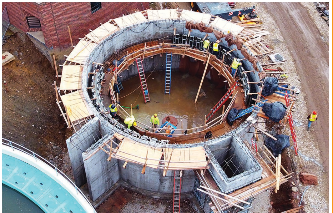
Meets strict EPA standards: This perspective gives an idea of the massive dimensions of one of the Peirce Island treatment tanks that now help treat an average of 6.1 million gallons of wastewater daily.
