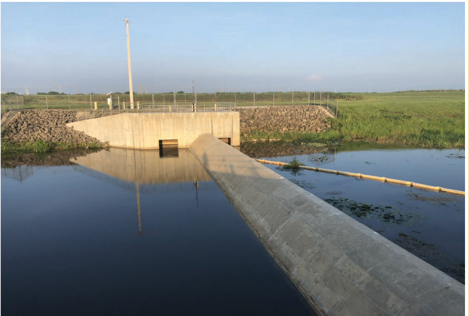
Protected by PENETRON: The concrete water flow control structure is downstream from the St. Lucie River (C-44) reservoir pump station.
