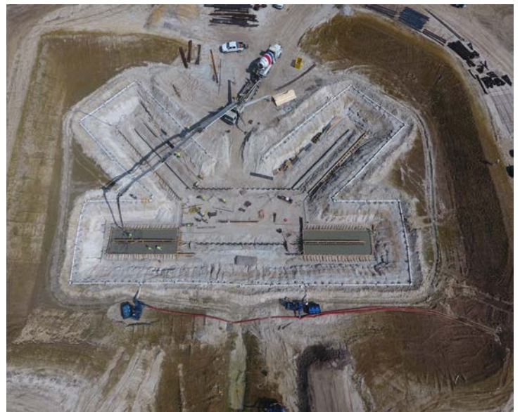
Under construction: An aerial view of the foundation of the massive pump station (C-43) for the St. Lucie River reservoir.
