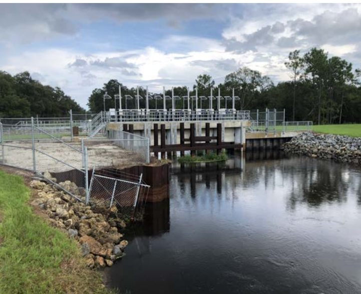
In the Kissimmee Chain of Lakes: This concrete control structure is located between Lake Rosalie and Lake Kissimmee (G-103).
